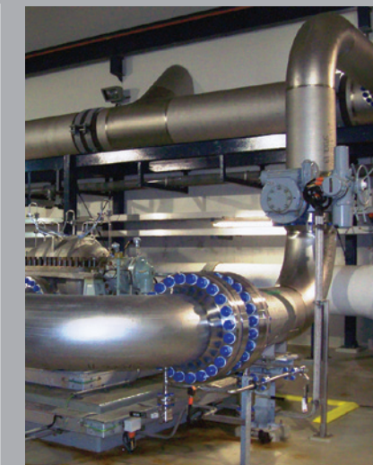
High pressure, super duplex stainless steel pipework at the seawater reverse osmosis (SWRO) desalination plant in Queensland, Australia. Duplex and super duplex stainless steels are default materials for the high pressure pipework in most RO plants worldwide due to their combination of high strength and excellent corrosion resistance.
